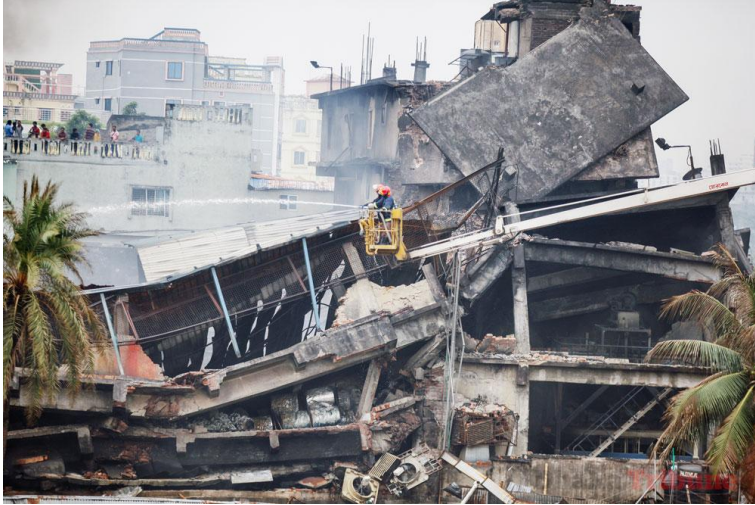
Fig4.8: Tampaco after fire hazard.
