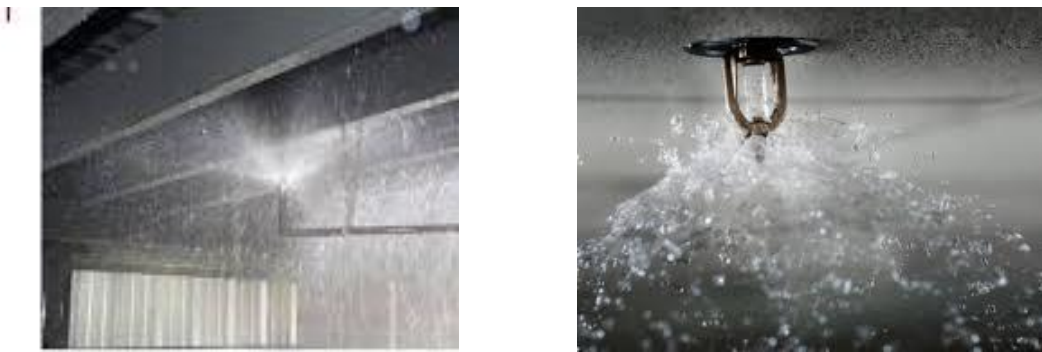
Fig 2.16: Automatic Sprinkler system.
