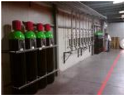
Fig 2.19: Gas extinguishing system
