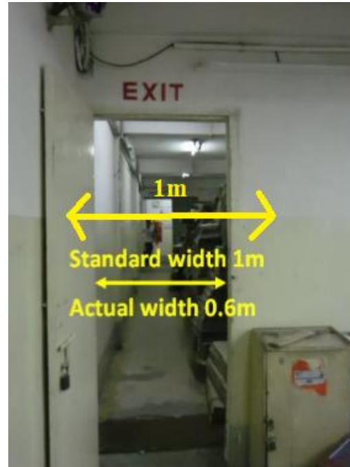
Figure-2.3: Hard factors: Exit door does not meet regulations.
