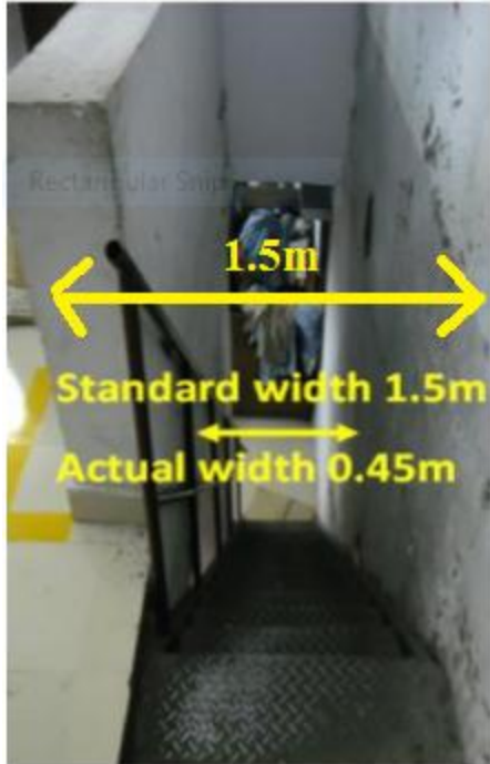
Figure-2.2: Hard factors: Stairway does not Meet regulations.
