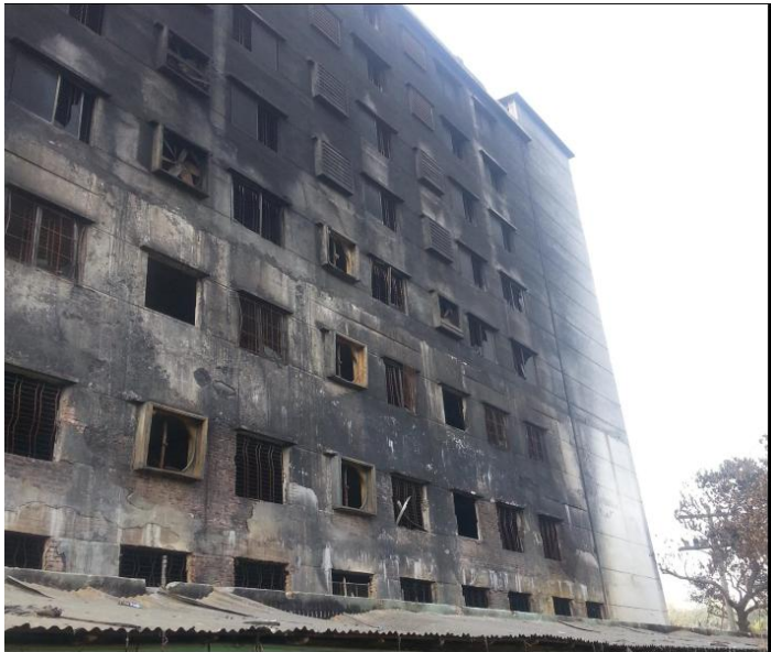
Fig 4.2: Tazreen Fashion ltd. status after the fire hazard
